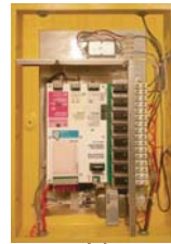
Douglas Satellite Panel installed near loads
