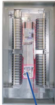
Central Lighting Control Relay Panel
